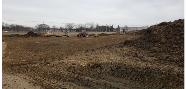
Soil modification typically adds lime or LKD to speed up the soil drying process.
