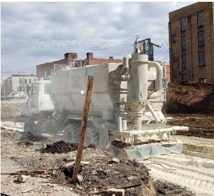
The option to use soil stabilization is limited due to current cement shortages.
